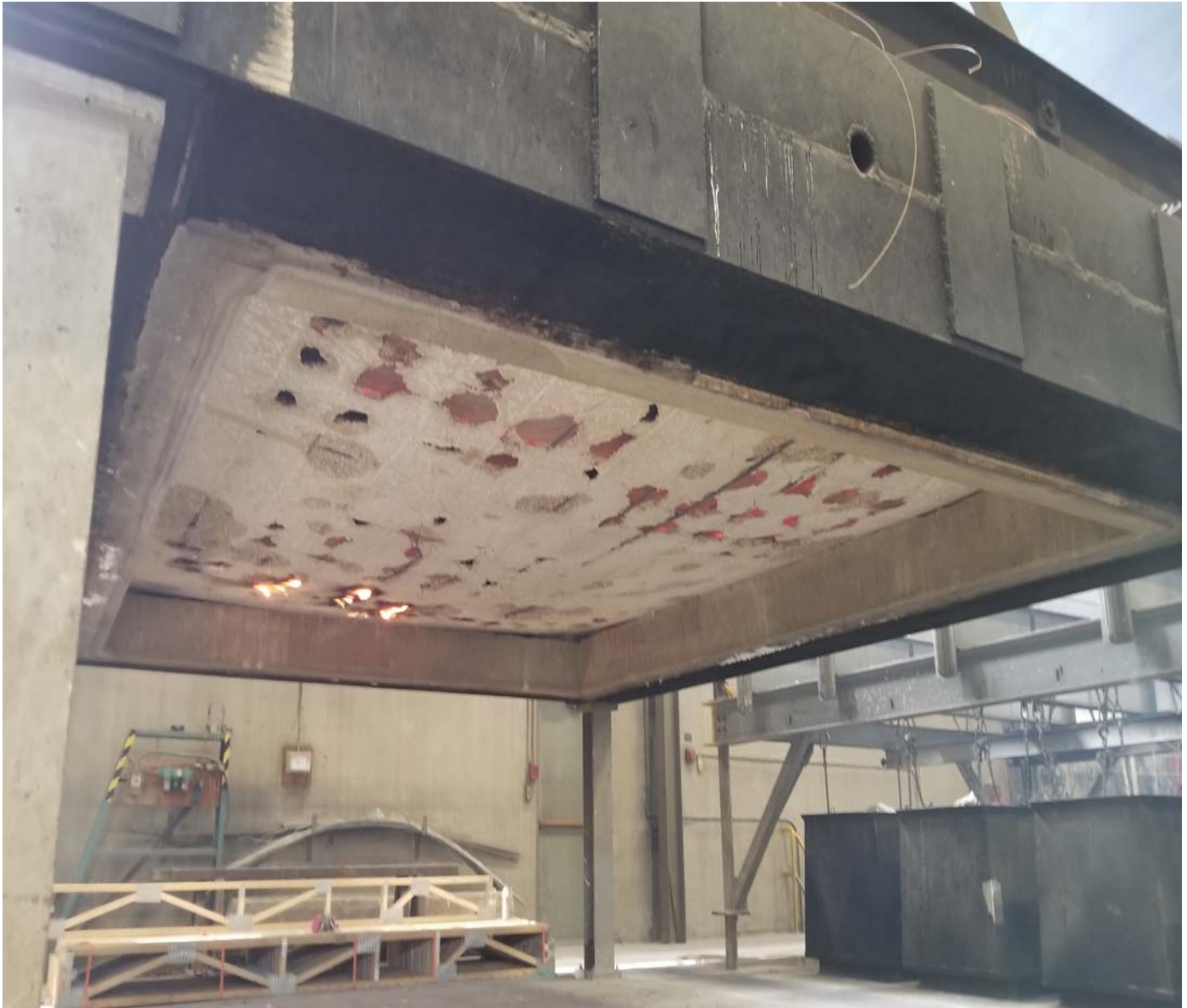
Figure 11 – Underside of test assembly after fire testing.
